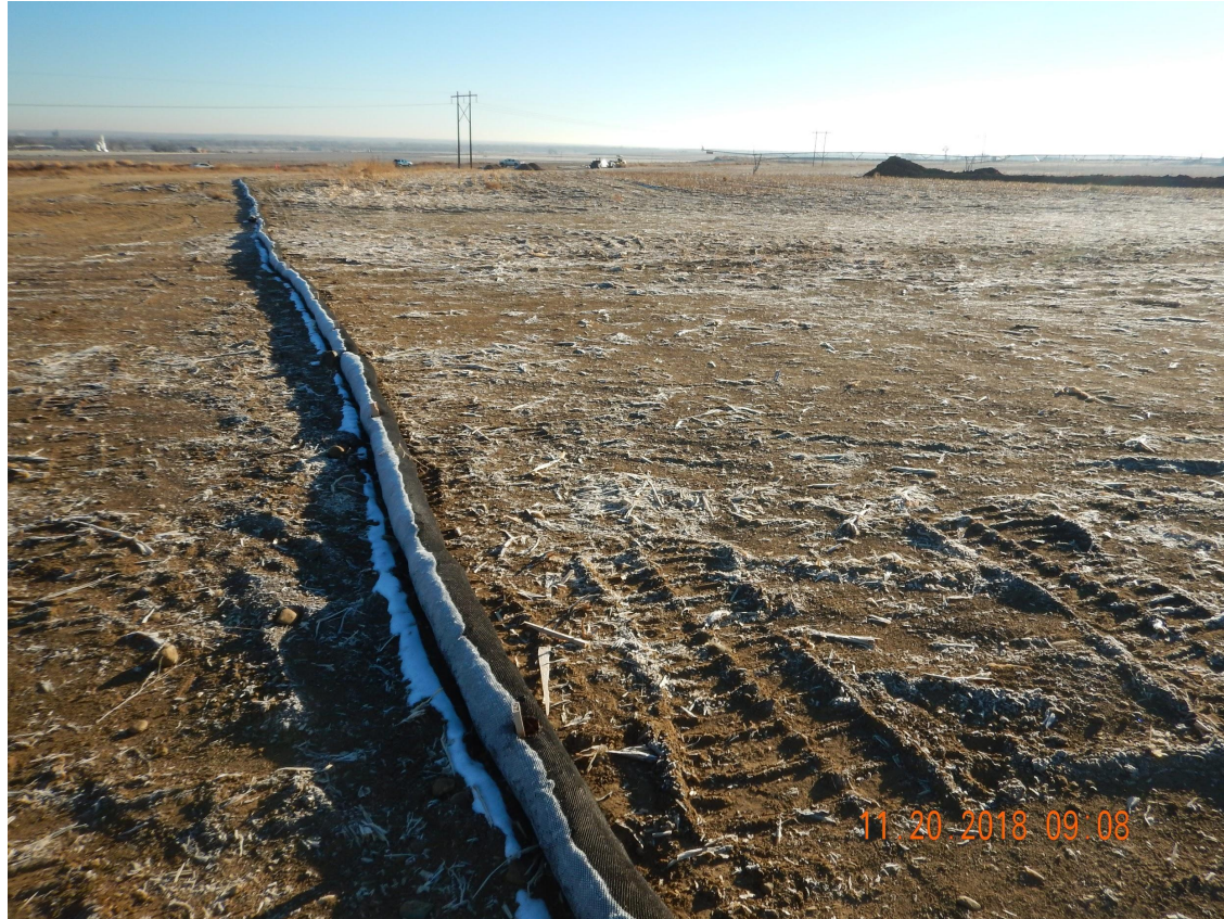
Photo 2. Photo taken from the northern perimeter of the location, facing East. Photo illustrates a temporary stormwater BMP which has been installed around the entire perimeter of the location. Filtrex wattle has been staked and trenched.
