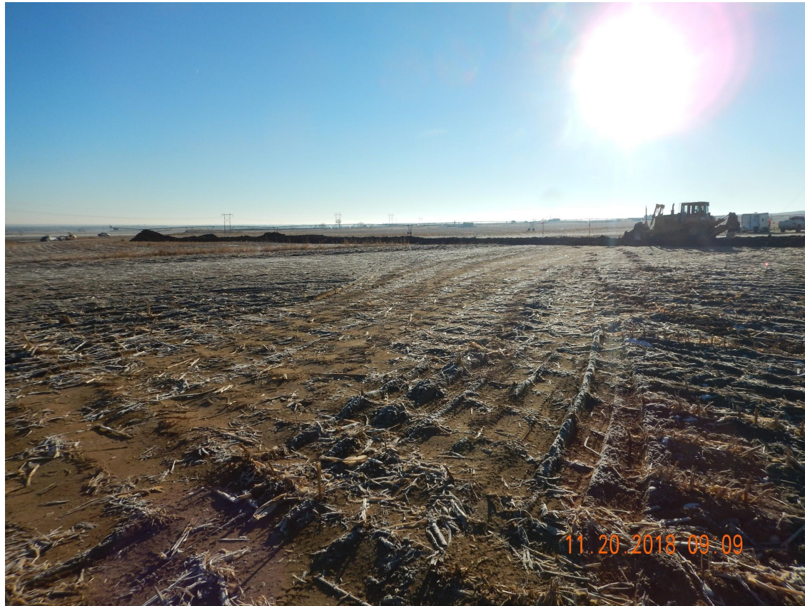
Photo 1. Photo taken from the northern location, facing South. Photo illustrates the start of topsoil salvage operations.
