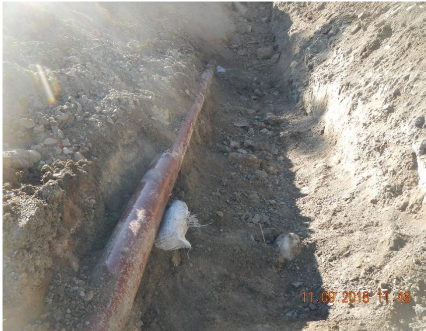
Failure points located above sandbags.
