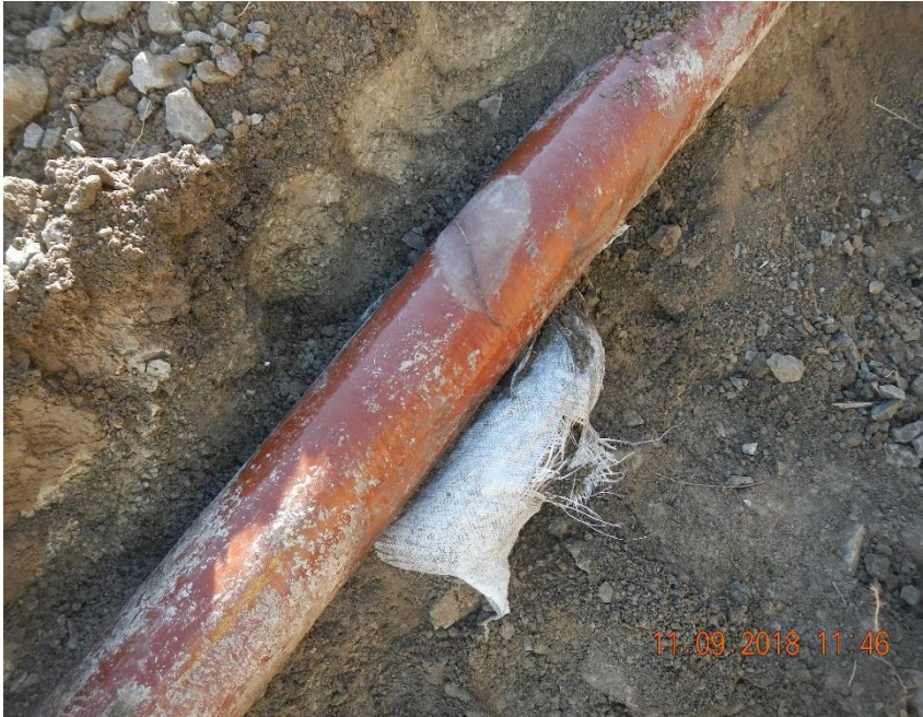
Downstream failure of fiberglass line.
