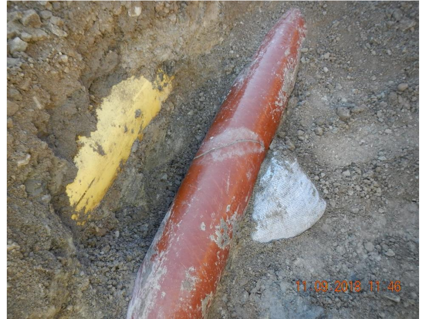
Upstream failure of fiberglass line. Abandoned steel gathering line in left of photo.
