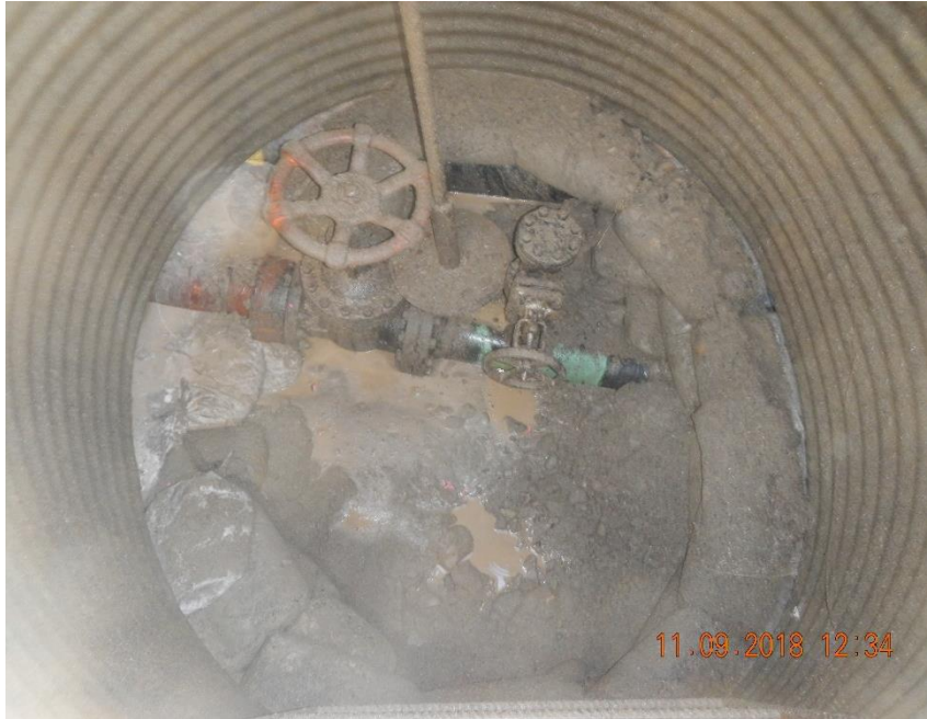
Valve can upstream of release point.
