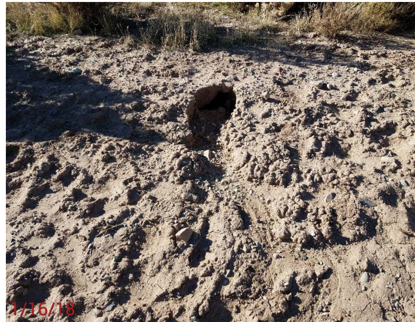
Location Photo #2, Hole in berm south end of separators.
