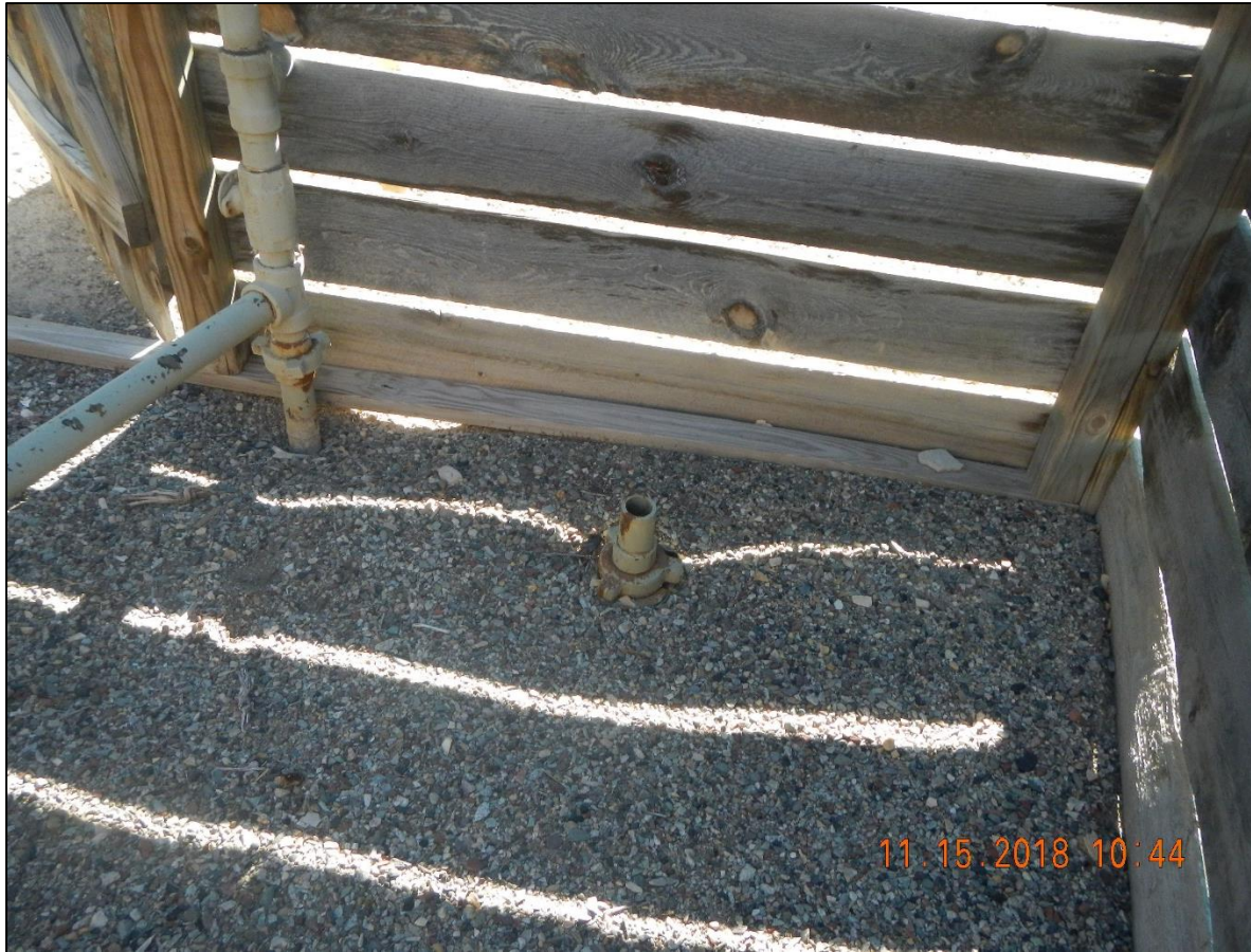
Unused equipment. Flowline riser is not LO/TO or marked.
