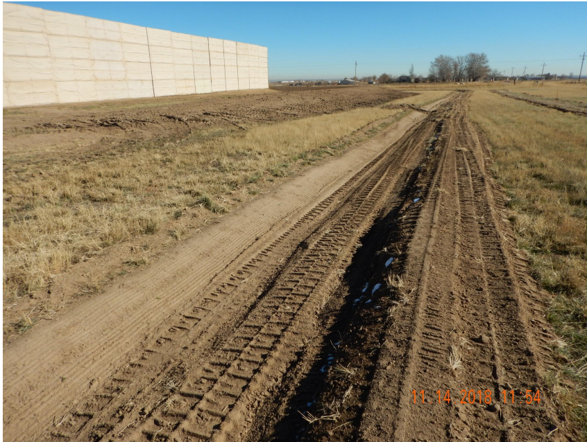
Photo 1. Photo taken from the southern perimeter of the location, facing East. Photo illustrates a ditch and berm BMP that has been installed around the entire perimeter of the location in conjunction with other BMPs.
