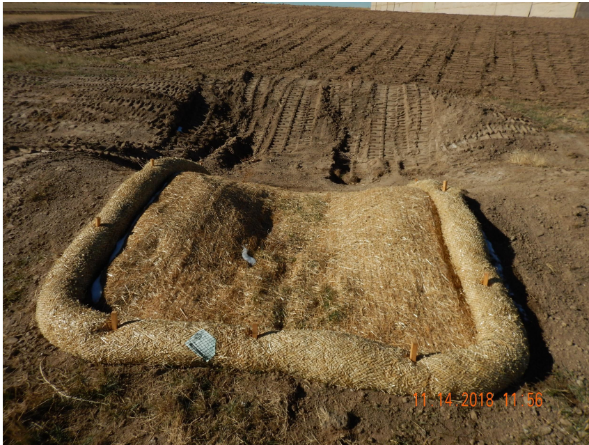
Photo 5. Photo taken from the eastern perimeter of the location, facing Southwest. Photo illustrates a sediment trap with a temporarily stabilized outlet. Also, photo illustrates the topsoil stockpile which has been temporarily stabilized with equipment tracking.
