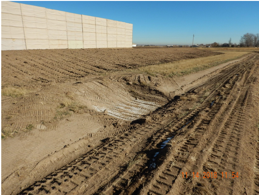
Photo 3. Photo taken from the southern perimeter of the location, facing Northeast. Photo illustrates the topsoil stockpile which has been temporarily stabilized with equipment tracking. Also, a retention area in conjunction with the ditch and berm BMP has been installed.
