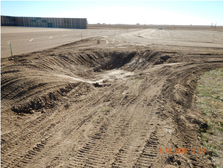
Photo 9. Photo taken from the northern perimeter of the location, facing South. See comments under Photo 3. Also, photo illustrates pad areas stabilized with gravel.
