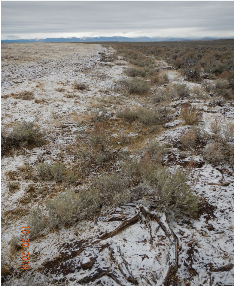
Photo#4: Remaining Perimeter ditches showing lack of complete re-contouring.
