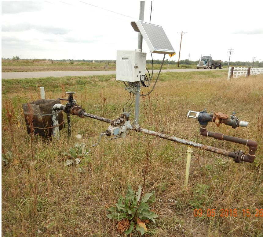
Photo 1. Photo taken from the eastern battery location on September 5, 2018. Photo illustrates the Operator failed to remove equipment after previous corrective actions were issued.
