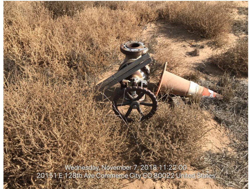
Photo#6 Unidentified Riser/Wellhead???
