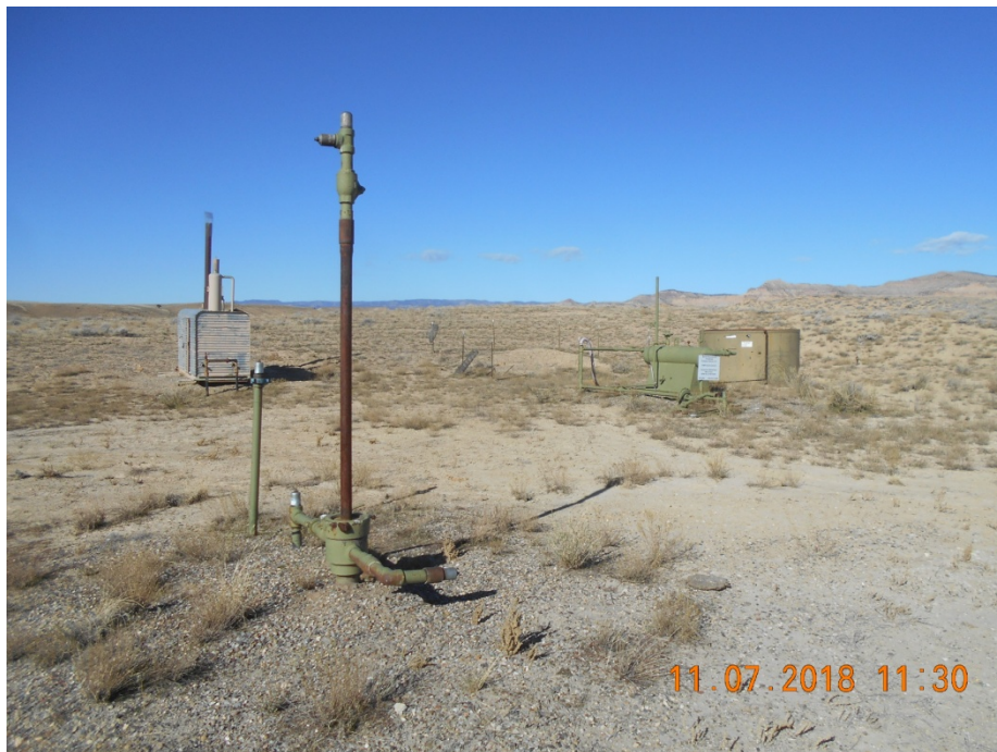
Wellhead with separators , tank and blowdown pit in background
