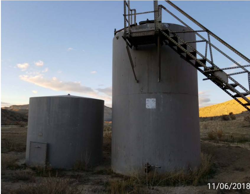
Tank battery looking northwest
