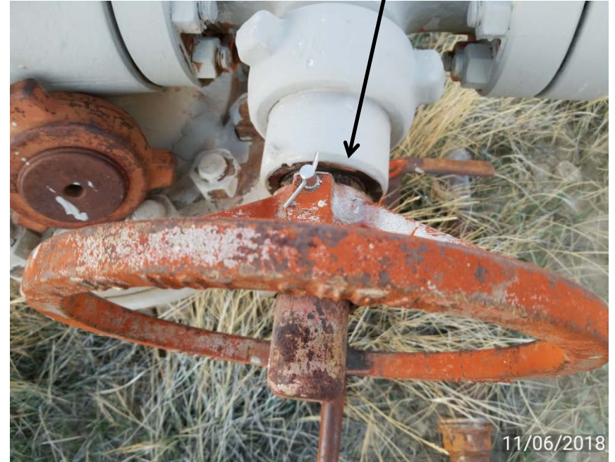
Gas leaking at casing valve
