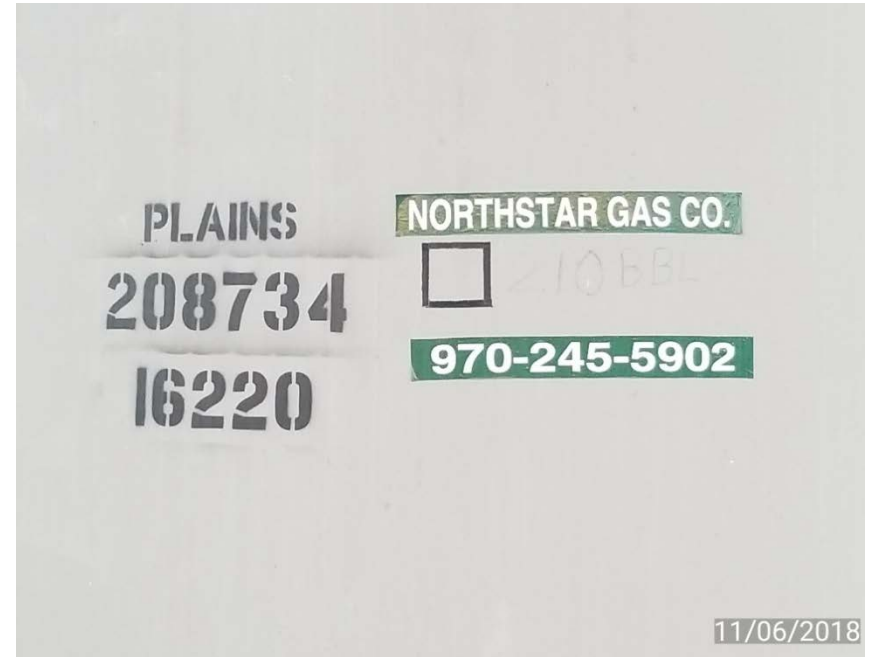
Tanks missing NFPA label and current phone number.
