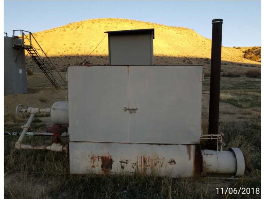
Gas leaking inside separator
