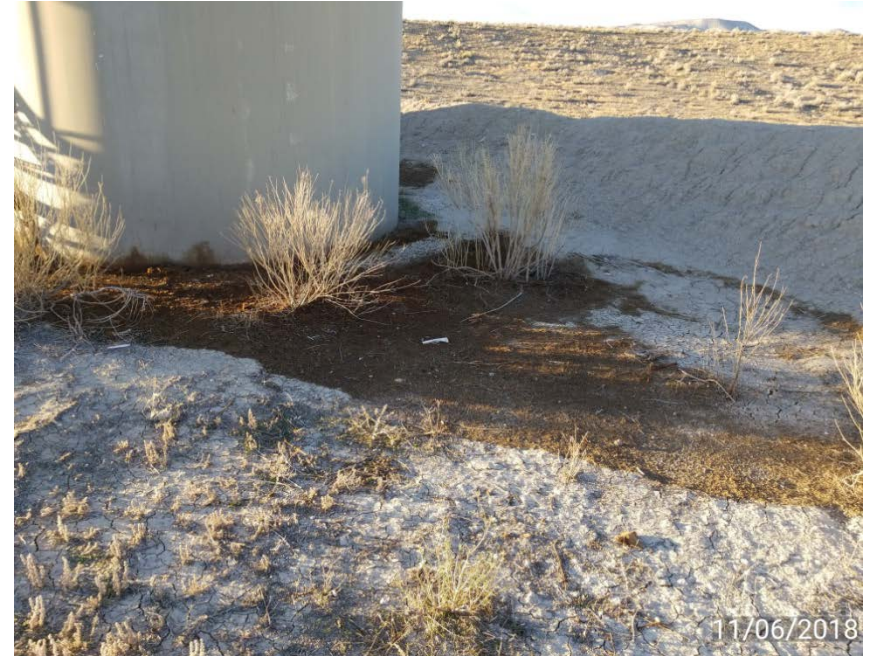
Condensate leaking from tank photo 1
