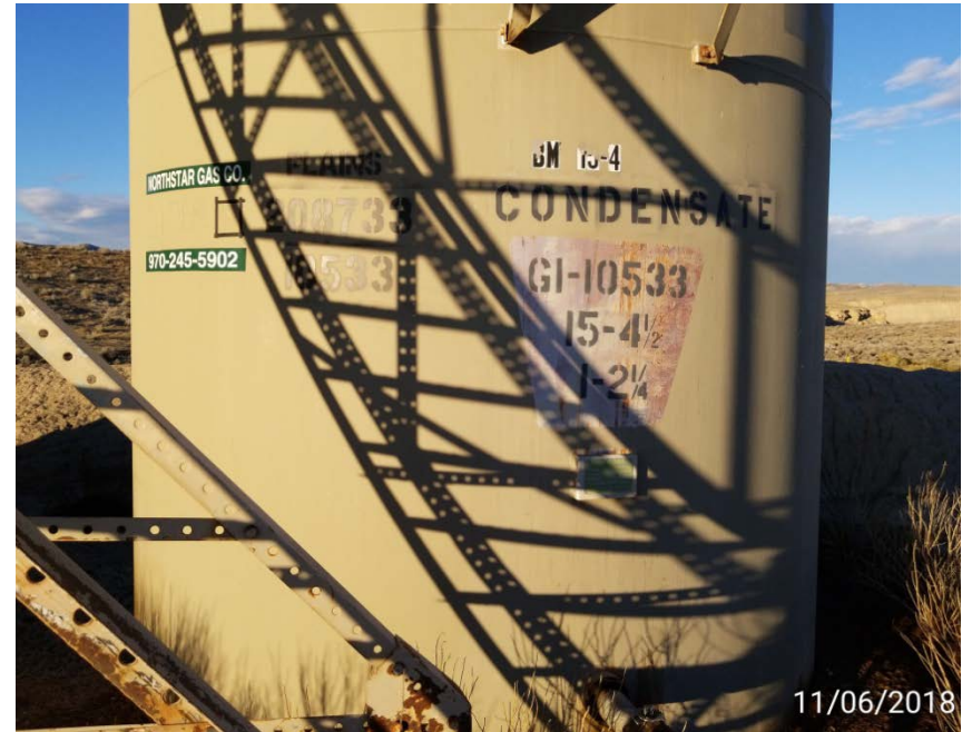
Tank missing NFPA label and current phone number
