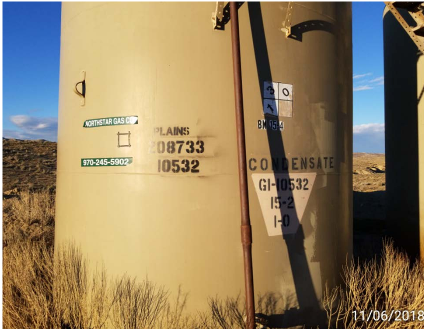
Tank missing NFPA label and current phone number
