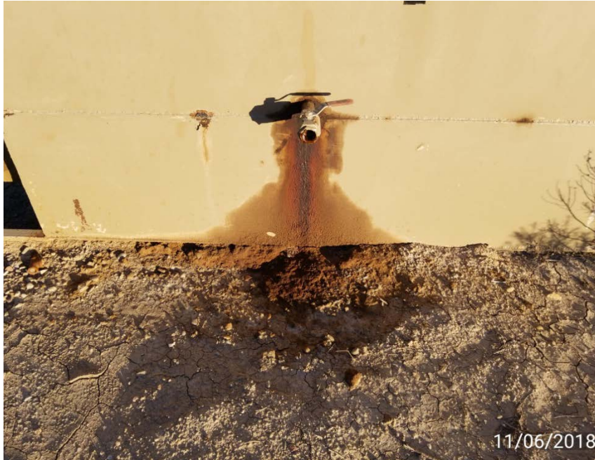
Separator had prior leak
