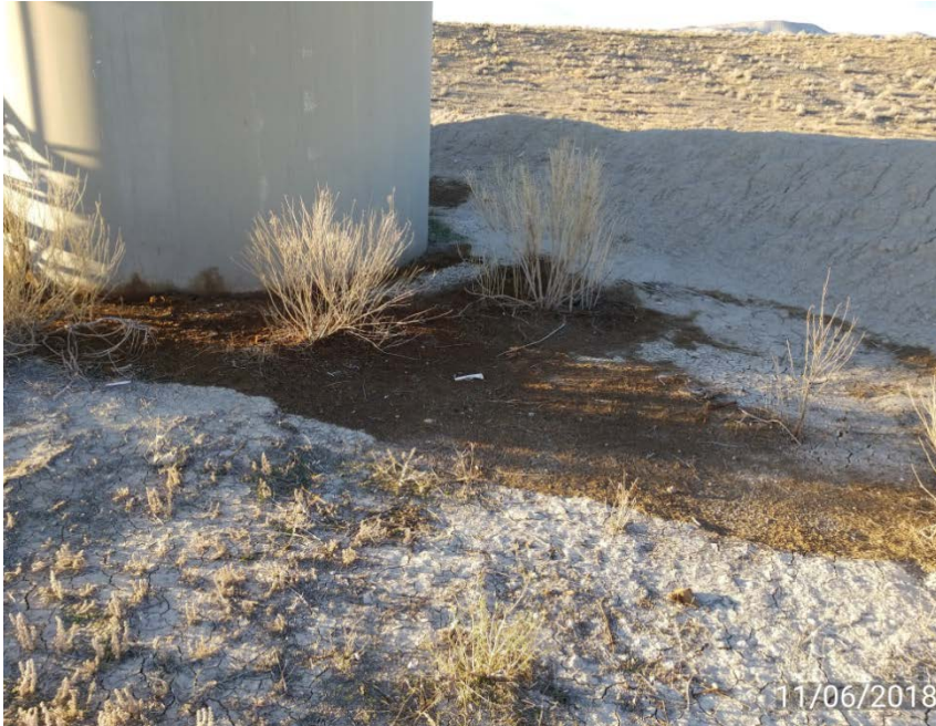
Condensate leaking from tank photo 2
