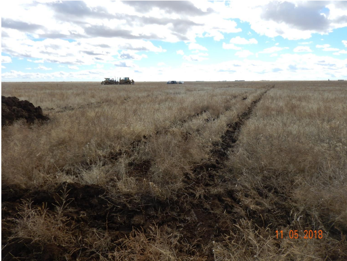
Photo 3: Photo taken from the northwest corner of the disturbance area, facing south. Photo shows construction in process. Photo also shows surface roughening has been used as a perimeter stormwater control
