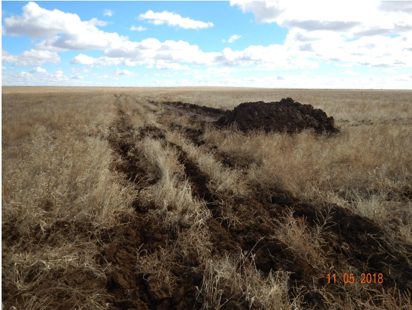
Photo 4: Photo taken from the northwest corner of the disturbance area, facing east. Photo shows construction in process. Photo also shows surface roughening has been used as a perimeter stormwater control
