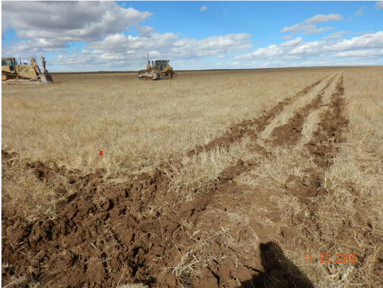
Photo 2: Photo taken from the southeast corner of the disturbance area, facing north. Photo shows construction in process. Photo also shows surface roughening has been used as a perimeter stormwater control
