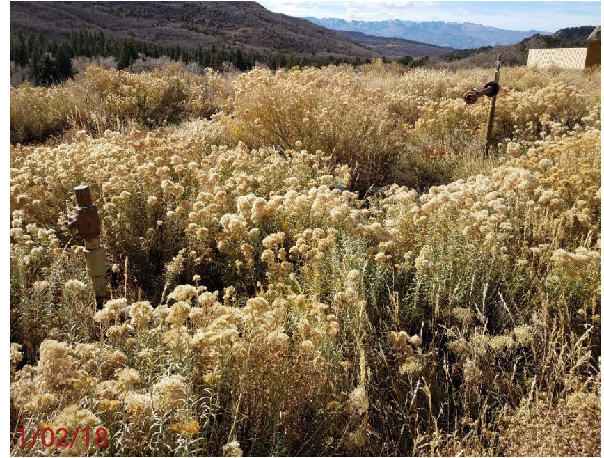
Location Photo #8, unmarked flowlines, unused equipment.
