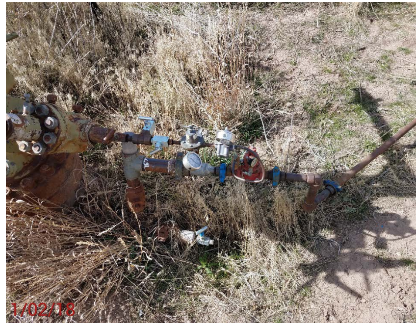
Location Photo #6, flow line coming from wellhead.
