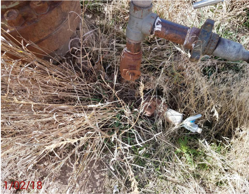
Location Photo #7 Flow line coming from wellhead plumbed into tank.
