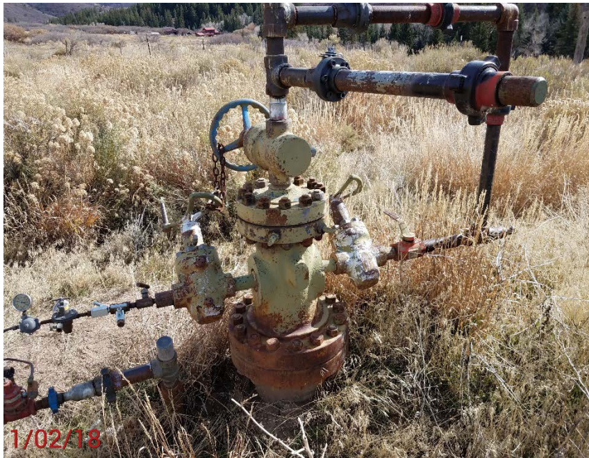
Location Photo #5, Missing wellhead sign
