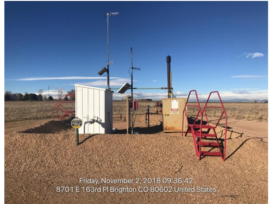
Photo#2 Separator/Gas Meter/Automation RTU
