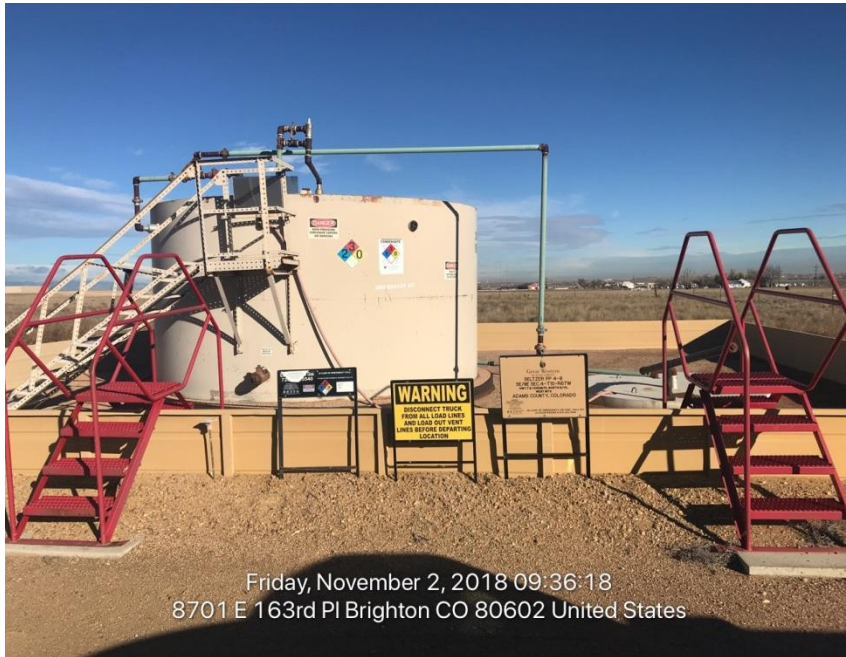
Photo#1 Production tank and Produced Water Pit
