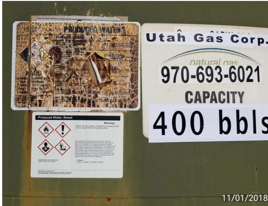
Produced water NFPA label unreadable on 1 tank
