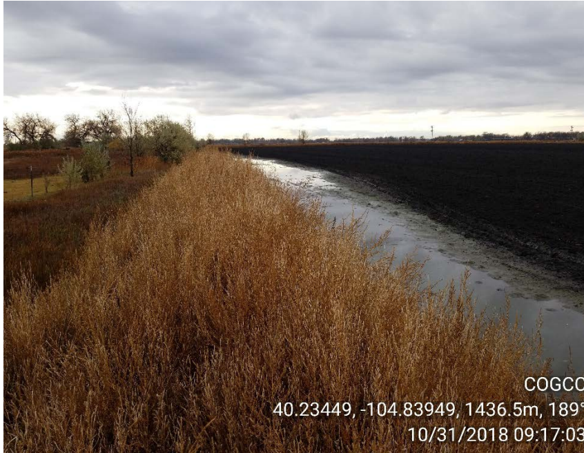
Photo 3 – Perimeter berm covered by weeds; Stormwater controls effective in keeping water/material on-site
