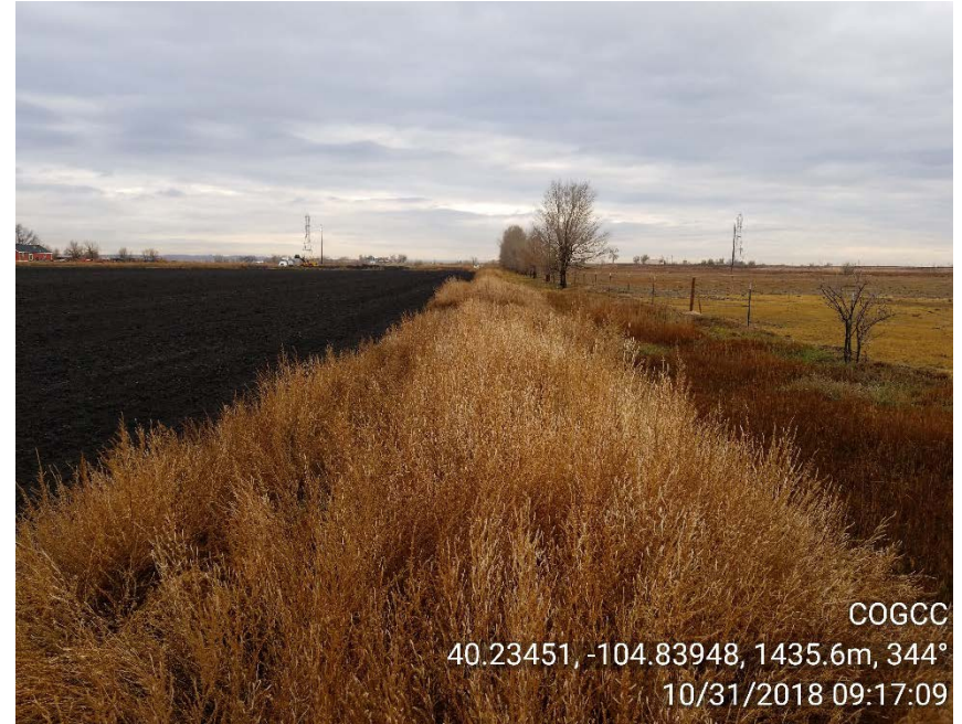
Photo 4 – Perimeter berm covered by weeds
