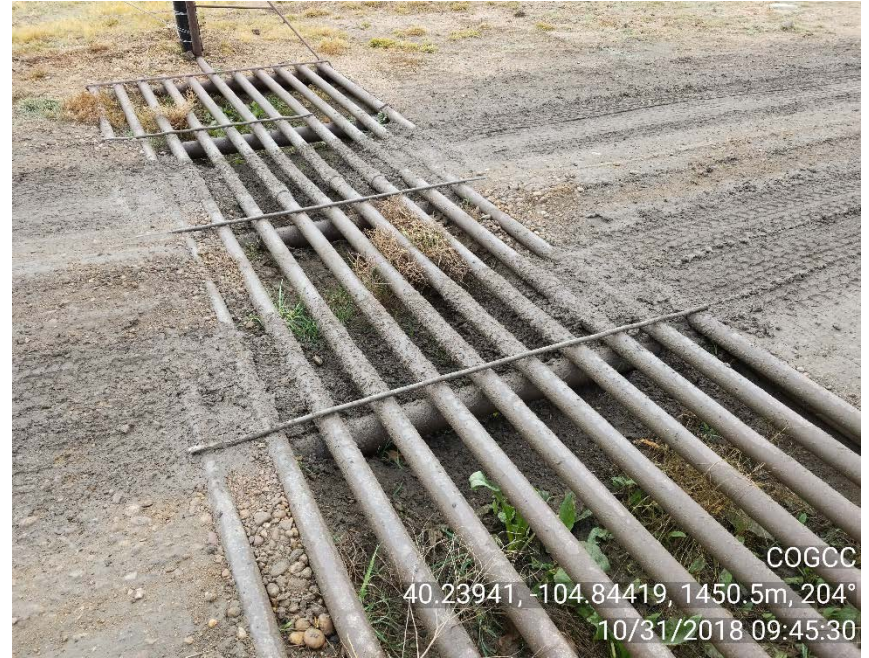
Photo 10 – Cattle guard on access road beginning to fill with bentonitic material
