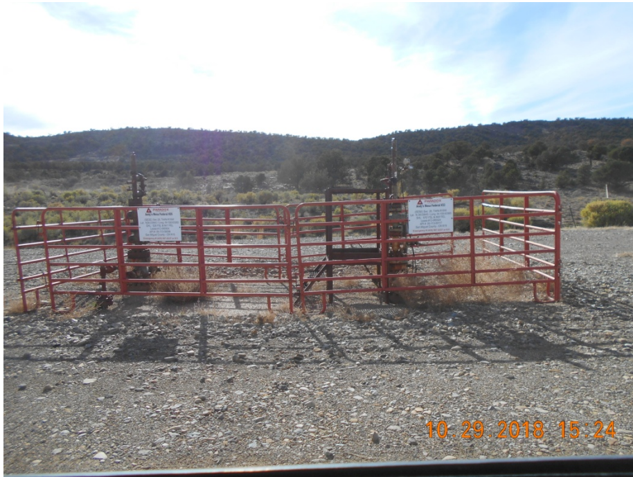
Wellhead with fence and sign
