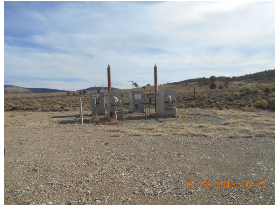
Separators and meter housings
