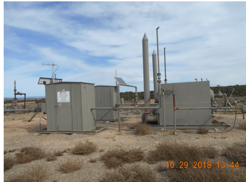
Separators and meter housing
