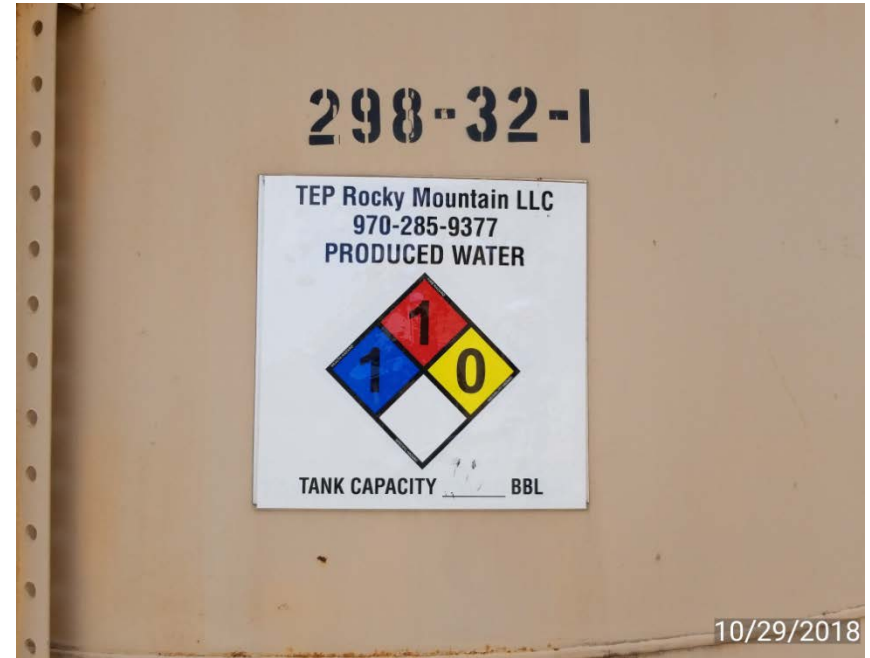
Tank capacity of "90" BBL no longer legible
