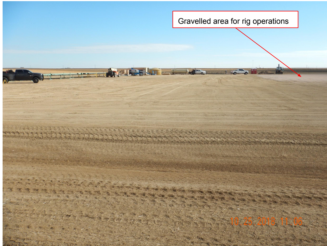
Photo 7. Photo taken from the northwestern perimeter of the location, facing East. Photo illustrates the northern well pad area which has been compacted but not necessarily stabilized from wind erosion. Operator shall ensure compliance with Rule 1002.e.(1) to reasonably control dust and minimize erosion which includes wind erosion.
