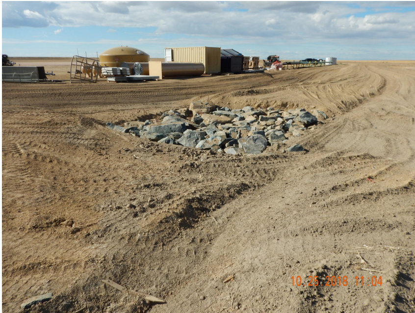
Photo 5. Photo taken from the northeast perimeter of the location, facing West. Operator has installed a sediment trap with a stabilized outlet.
