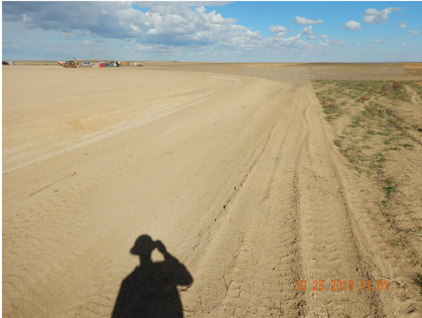
Photo 3. Photo taken from the eastern perimeter of the location, facing North. Operator has installed 2 sets of ditch and berm BMPs around the location.
