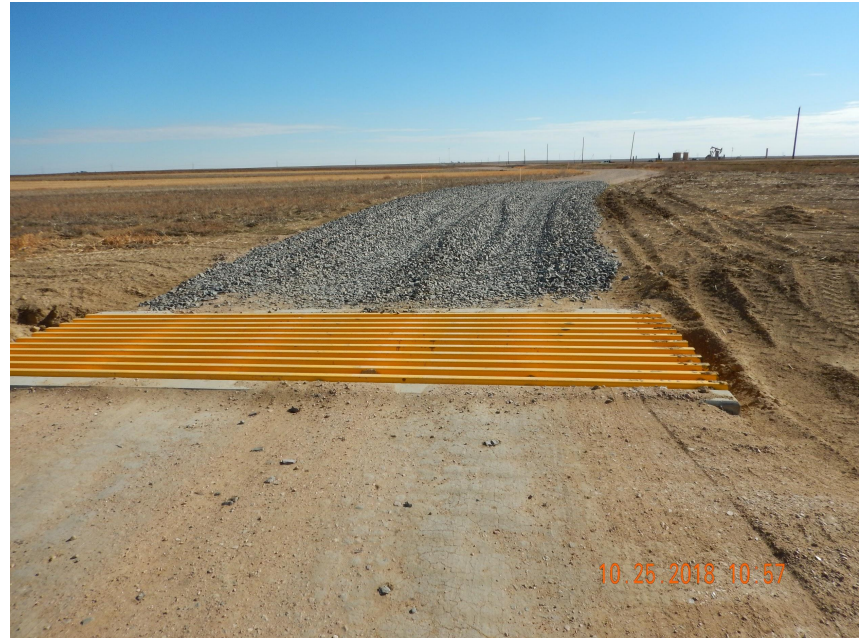
Photo 2. Photo taken from the entrance of the location, facing East. Operator has installed vehicle tracking devices which appear to be in proper functioning condition.
