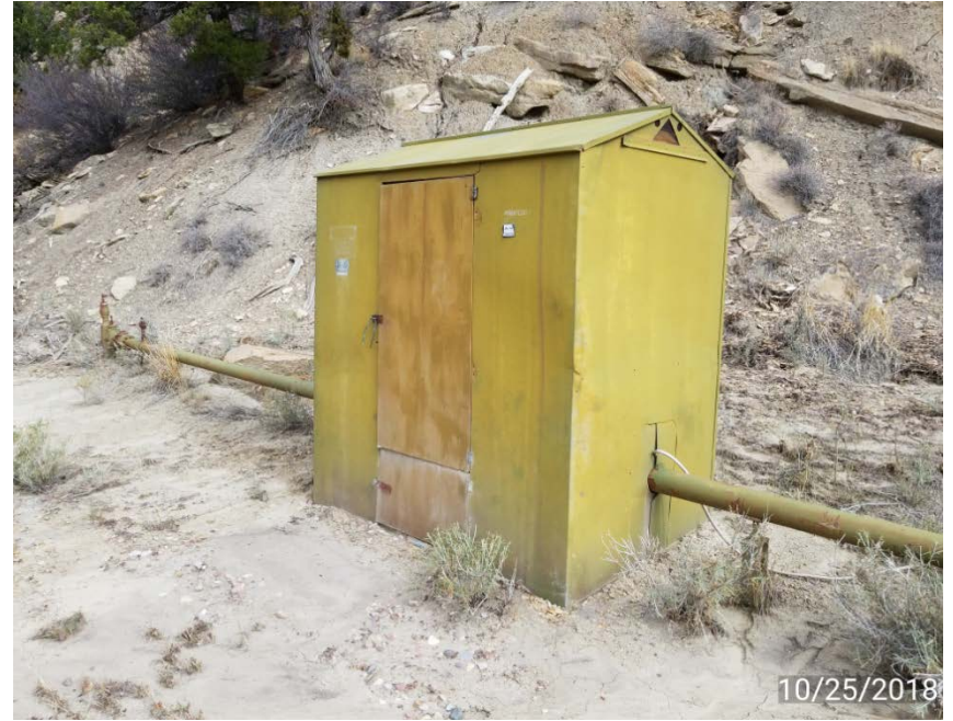
Gas meter building
