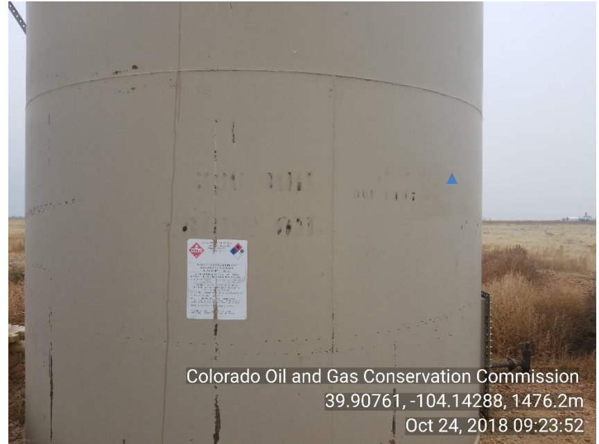
Photo 8 Tank volume and label not legible
