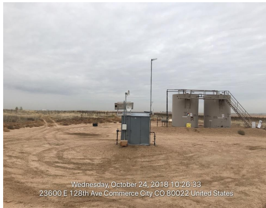
Photo#2 Gas meter and Production Tanks and Pit
