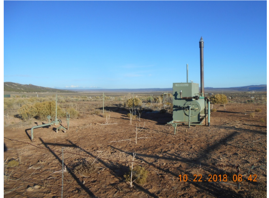
Separator with risers locked out/ tagged out
