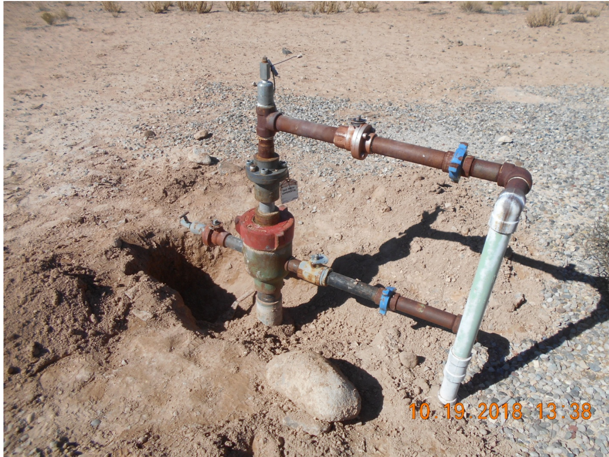
Wellhead with bradenhead valve exposed
