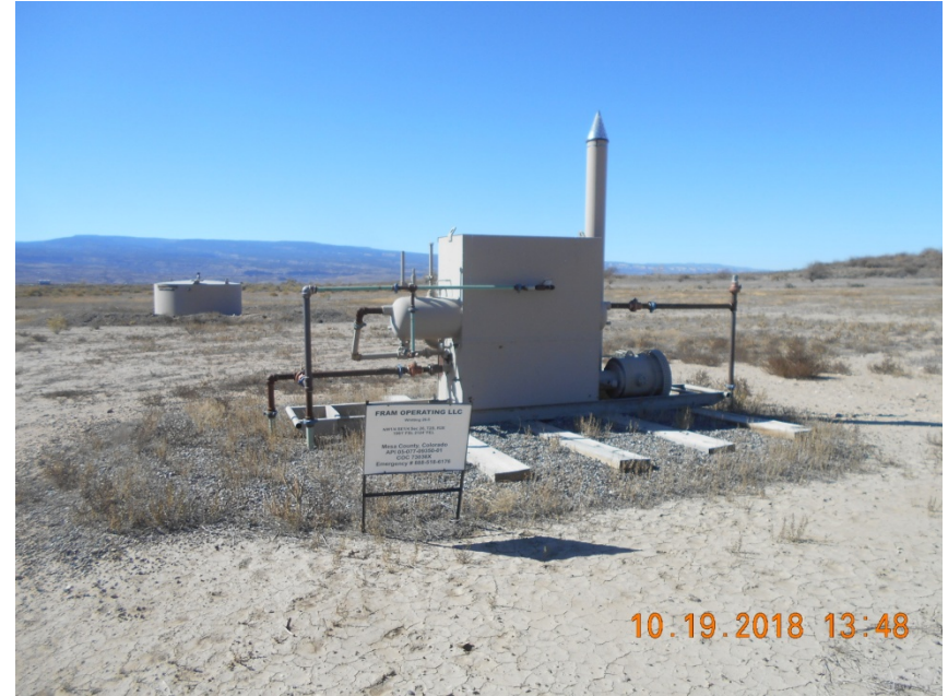
Separator with sign. Produced water tank in background. No NFPA labels or volumes posted.
