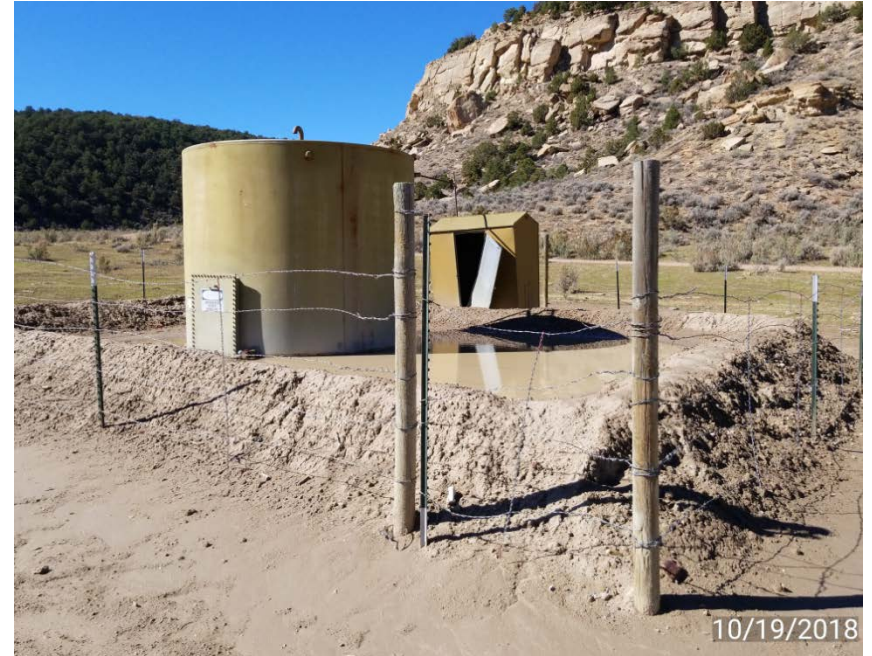
Tank on side of location. Belongs to Summit.
