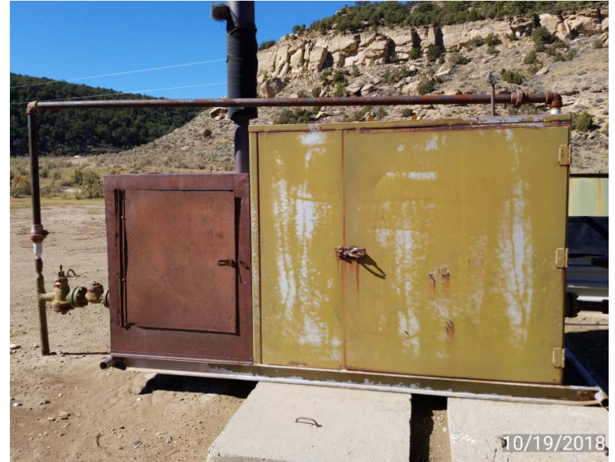
Small gas leak inside separator building
