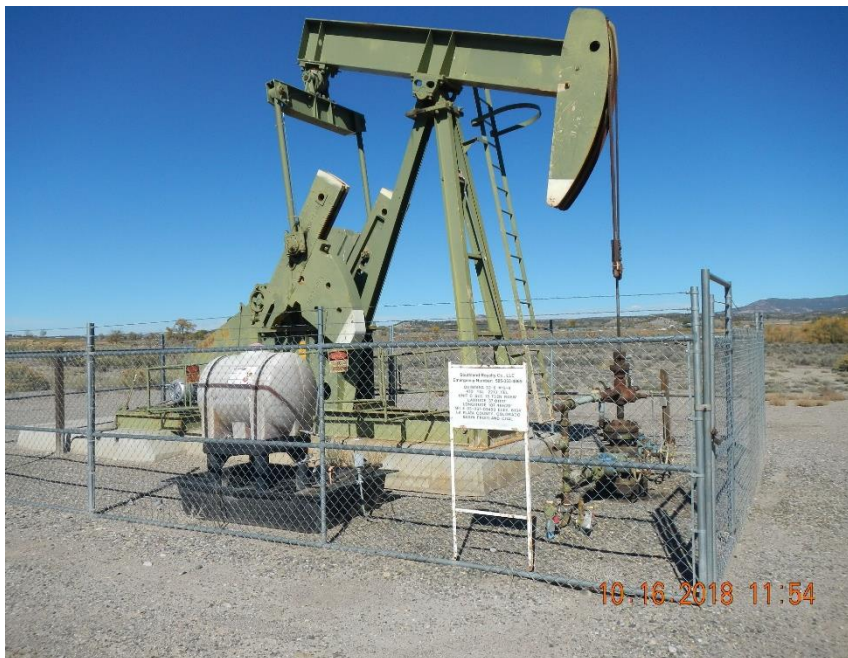
Secondary containment for chemical container at the #15-4.
