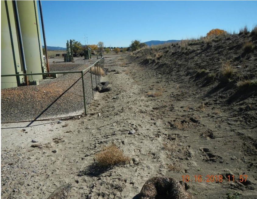
Perimeter berm is filling with sediment. Wattles are damaged and in disrepair.
