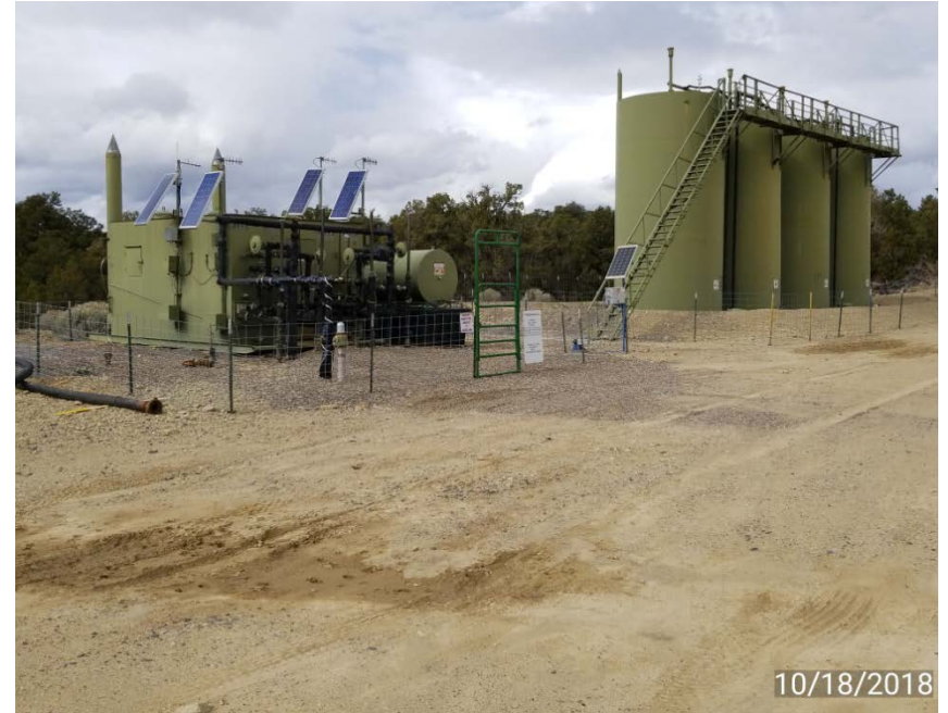
Location separator & tanks
