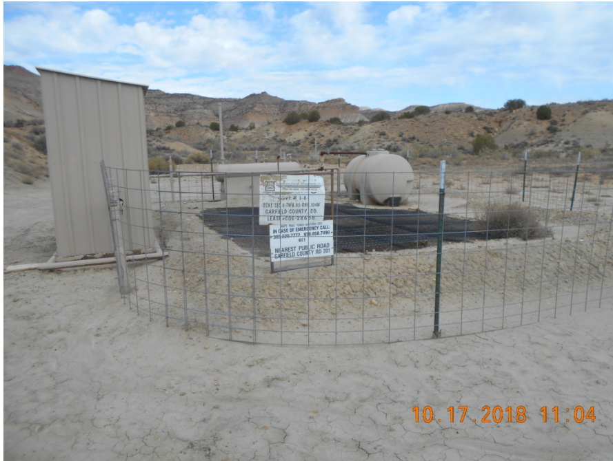
Separator, Meter housing and blowdown pit with fencing and sign
