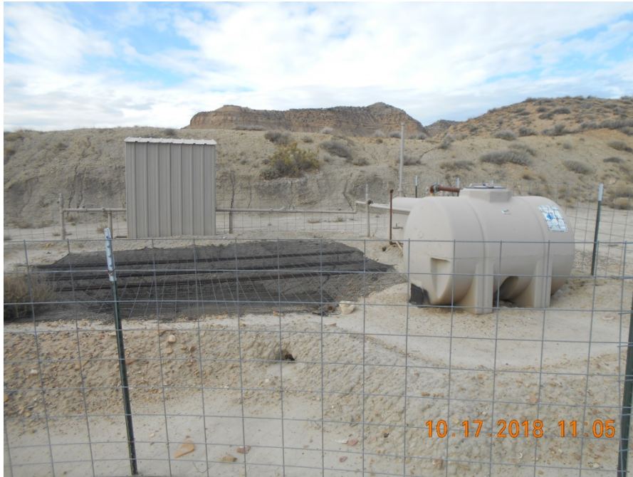
Separator, Meter housing and blowdown pit and tank with fencing and sign
