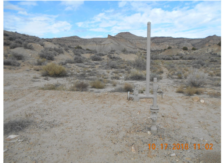
4" unused riser. Locked out/tagged out
