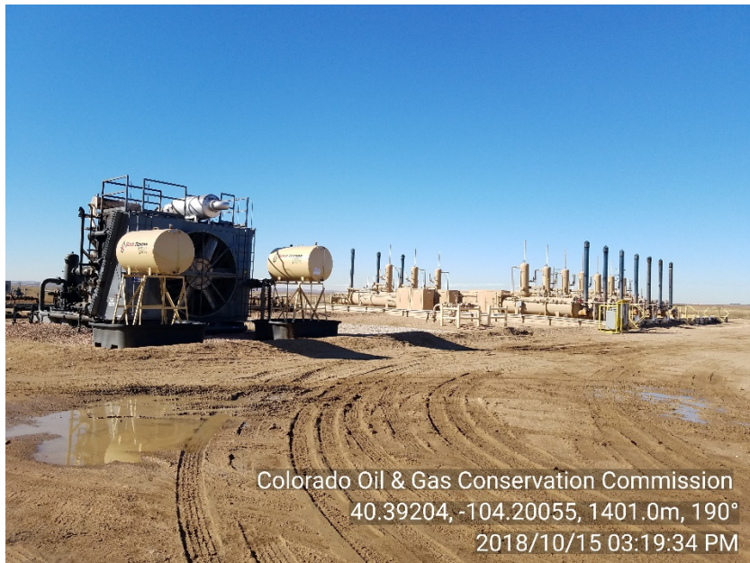
Photo #3 Pronghorn F-22 Pad & J-15 Pad Compressor & Separators
