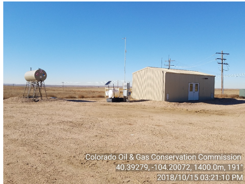
Photo #4 Pronghorn F-22 Pad & J-15 Pad Gas meter runs
