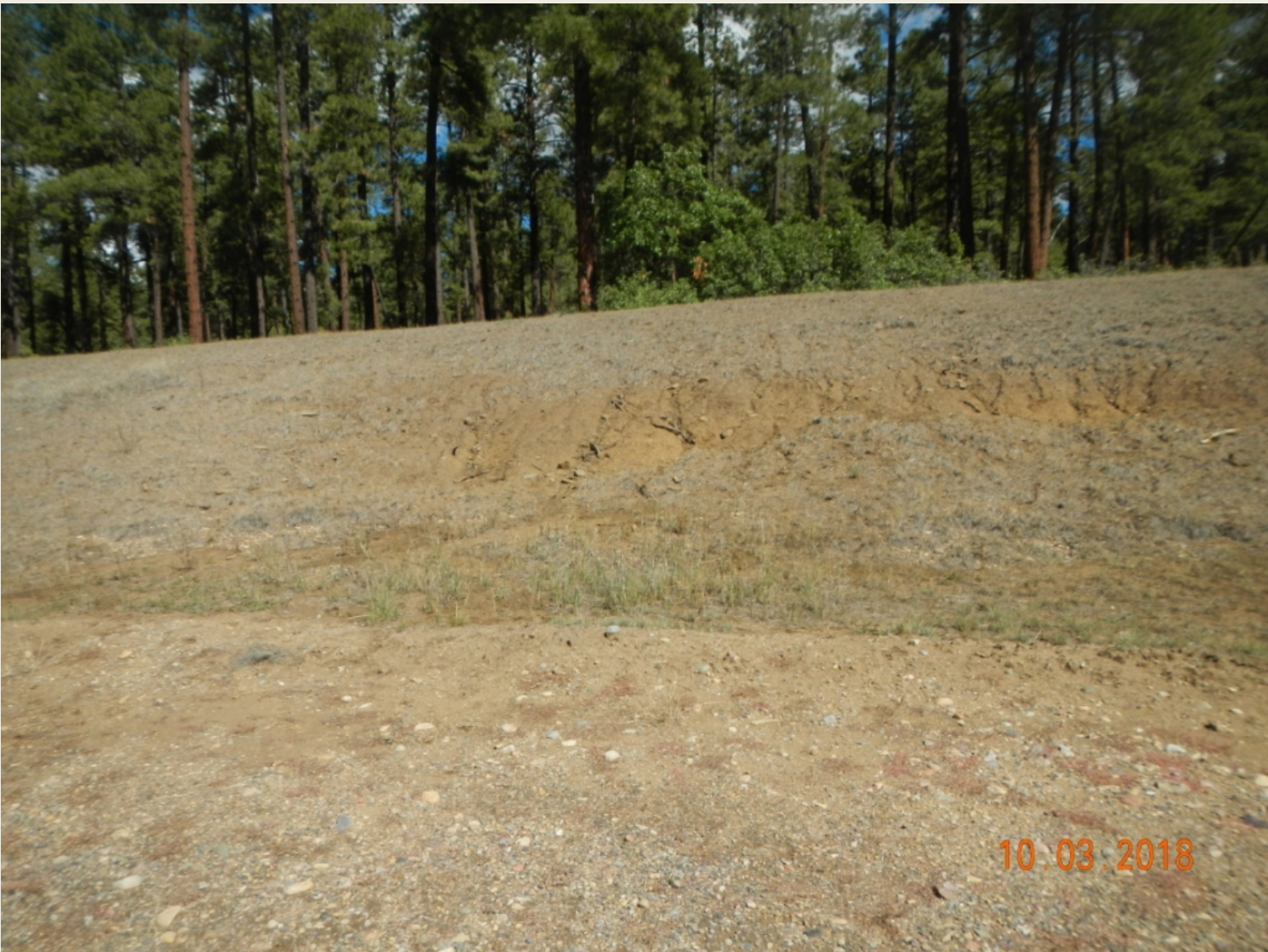
Photo 4. View of area in the eastern cut-slope where rilling is occurring on sparsely vegetated slope.
