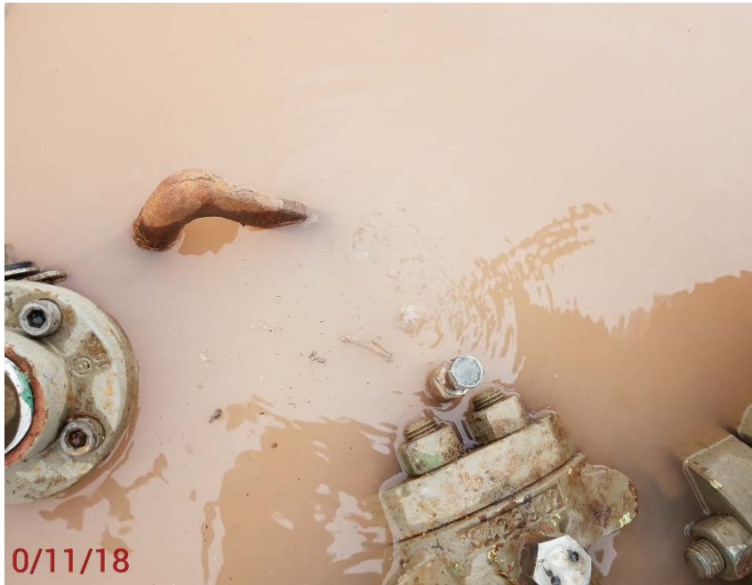
Location Photo #5, Leaking casing valve
