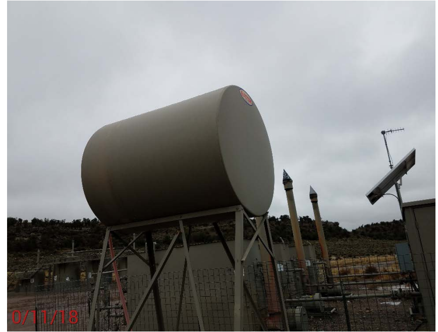
Location Photo #4, missing sign
