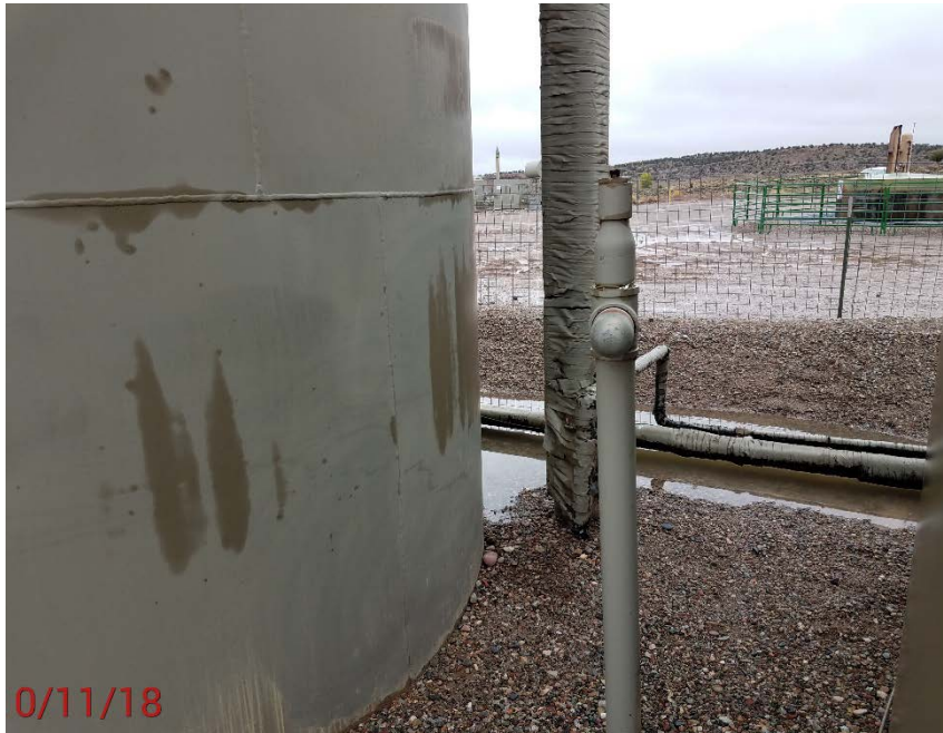
Location Photo #7, unused/unmarked flowline riser
