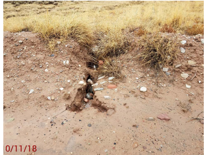
Location Photo #8, Storm water issue, sediment being moved off location.
