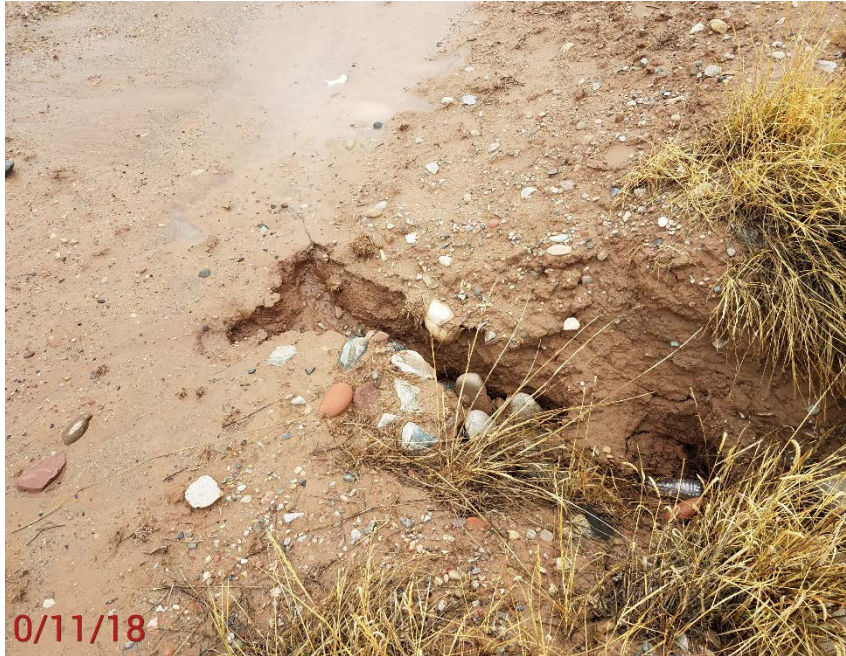
Location Photo #9, storm water issue, Sediment being moved from location
