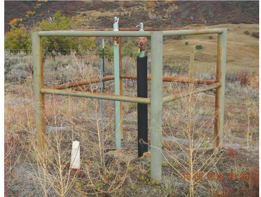
Both 2" valves are locked out in the closed position.
