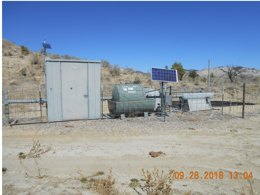
Separator and Meter Housing and blowdown pit
