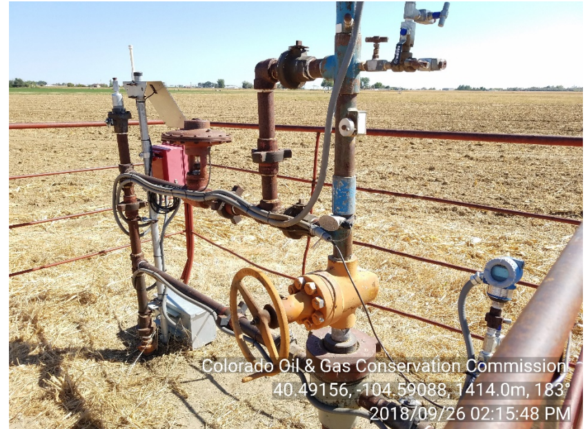
Photo #2 WPF III A18-2 wellhead Appears SI – valves shut
