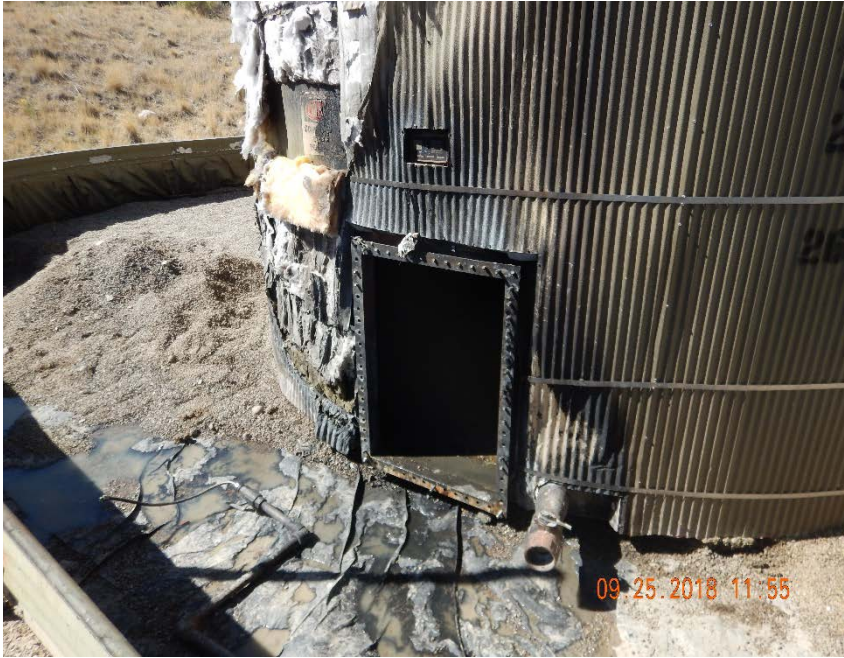
Photo #3 – View of impacted tank from NE corner.
