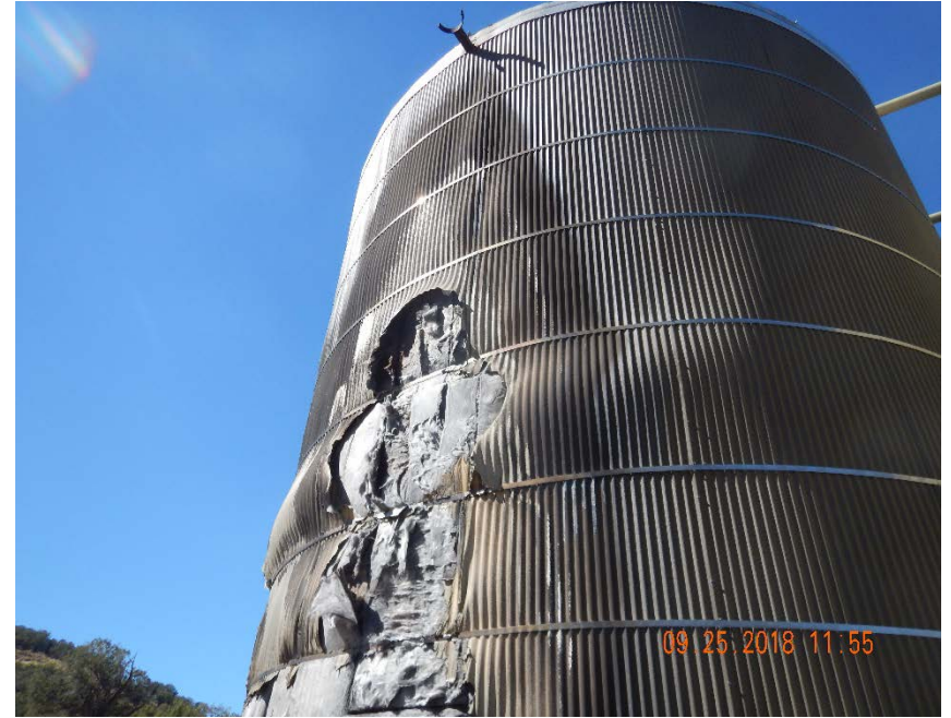
Photo #4 – Fire damage extending up the side of the impacted tank.
