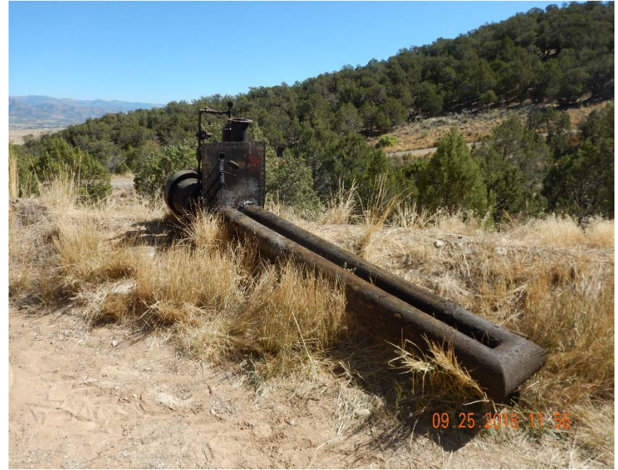
Photo #6 – Tank heater was pulled out of tank and being stored outside of tank battery berm on inspection date.
