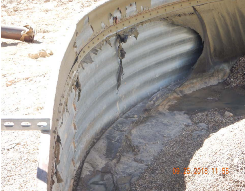
Photo #5 – Tank battery liner was compromised at SE corner due to fire damage.
