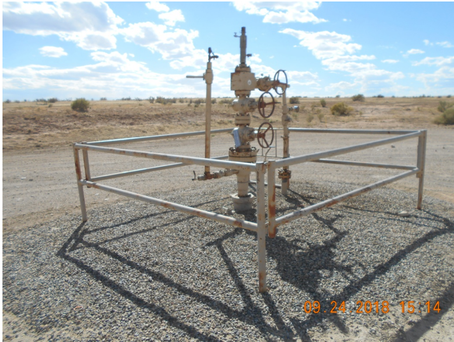
Wellhead with fencing
