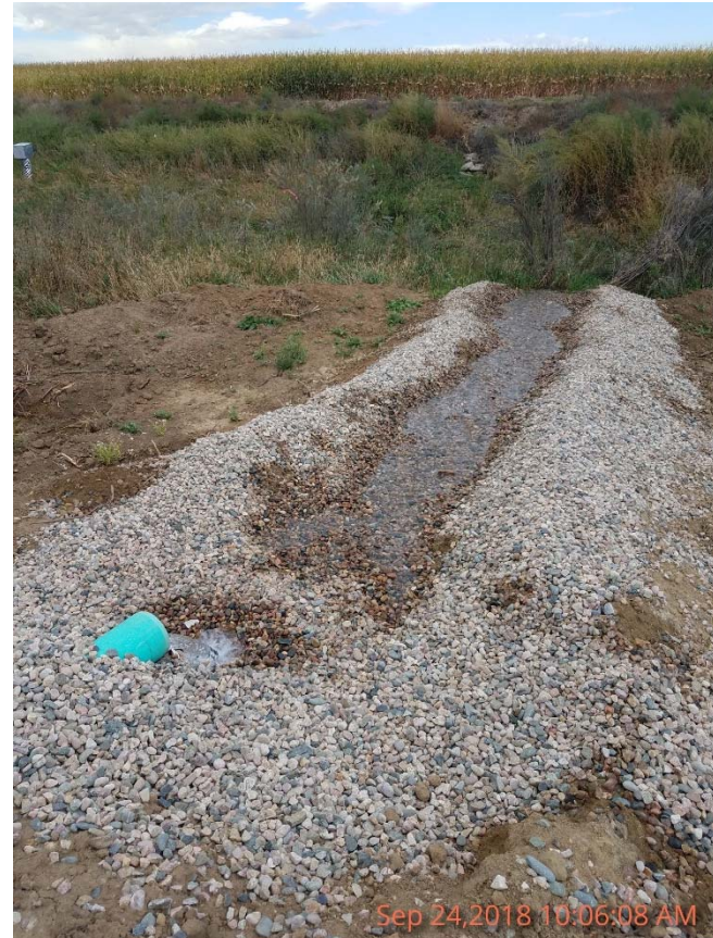
Photo 4 – View of outfall of groundwater drain installed on residential development property located adjacent and north (upgradient) of former tank battery.
