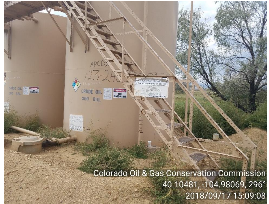
PHOTO #2: TANK BATTERY/WEEDS INSIDE BERMES
