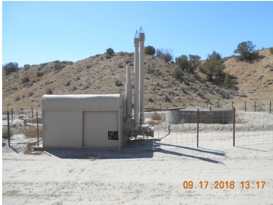
Separator and Tank battery with fencing .
