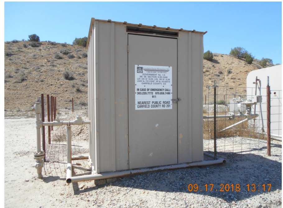
Meter housing with sign
