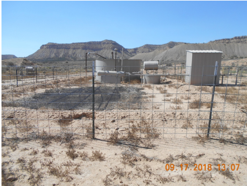
Separator, Meter housing and E. side blowdown pit.
