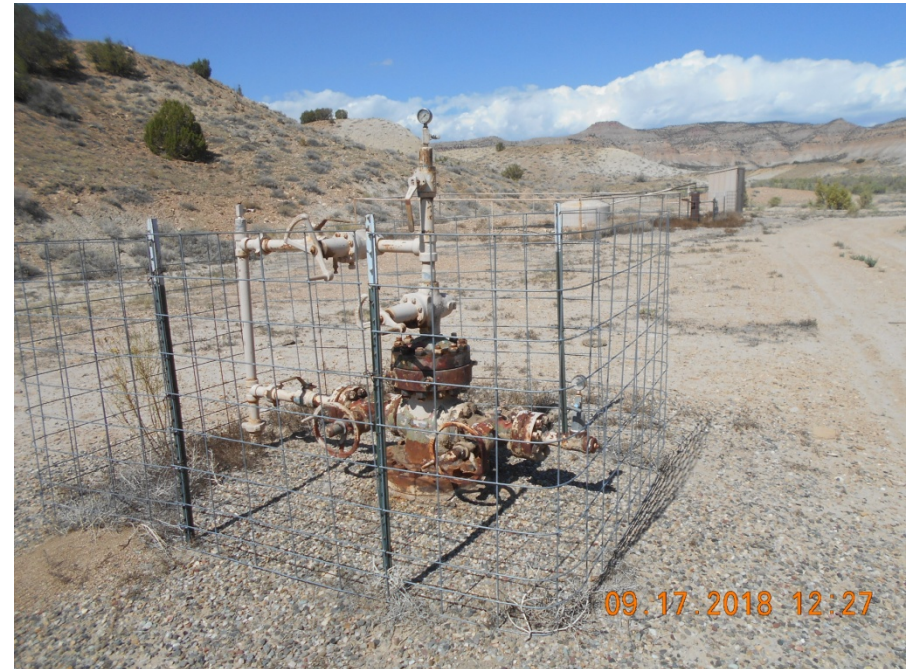
Wellhead with fencing
