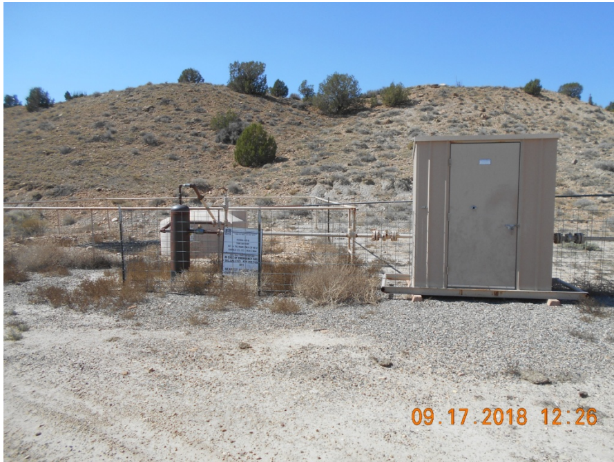
Meter housing and Tank battery with sign.
