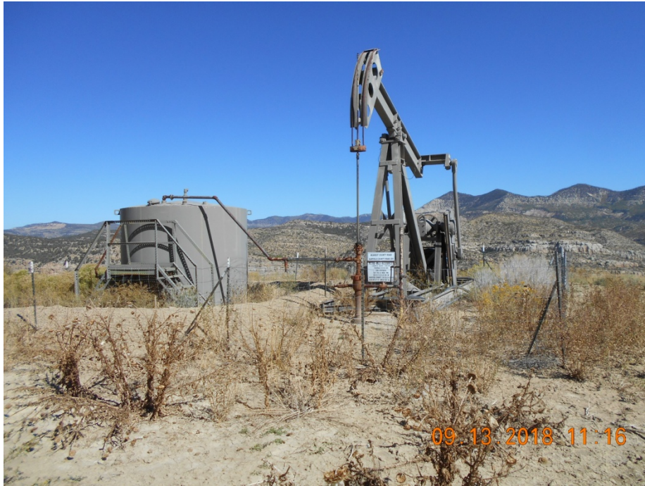
Pump jack and Tank battery
