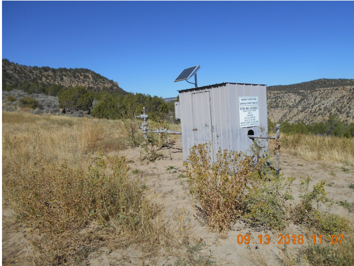
Wellhead and Meter Housing
