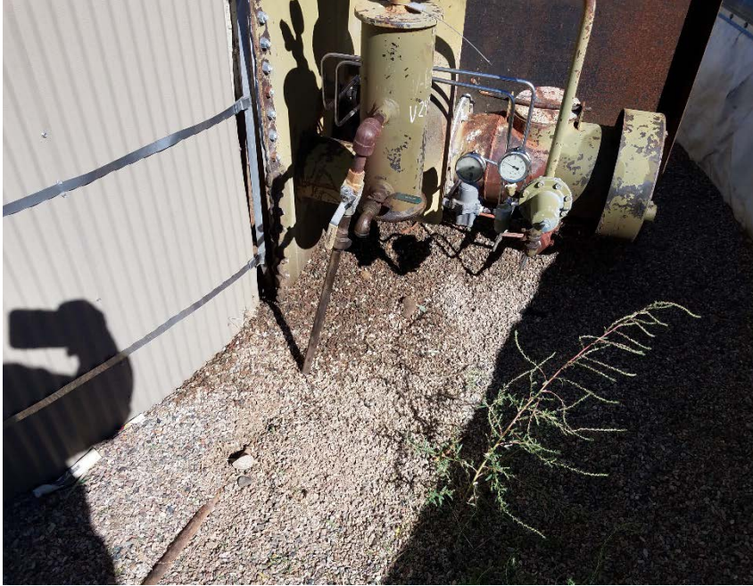
Location Photo #5, battery containment
