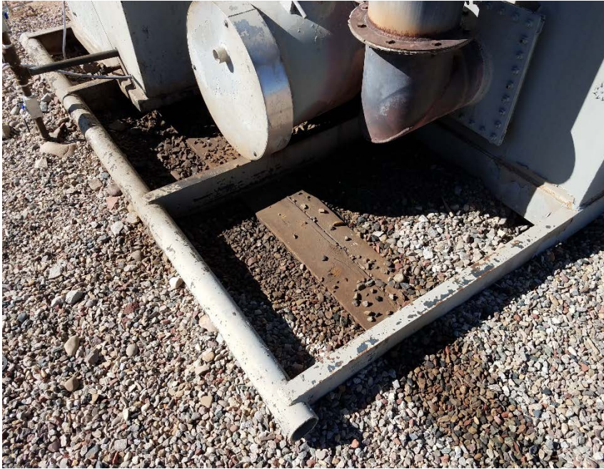
Location Photo #3, stained round near separator
