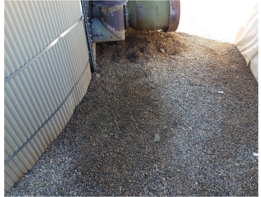
Location Photo #4, battery containment
