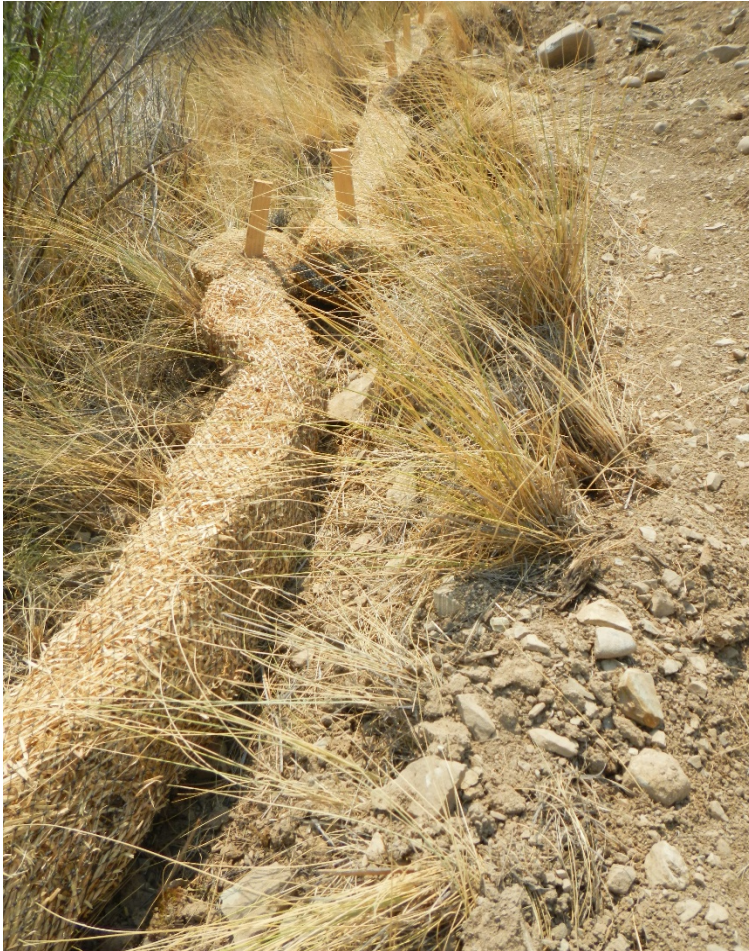
Photo#2: 8/14/18 Perimeter Wattles were not properly installed.
