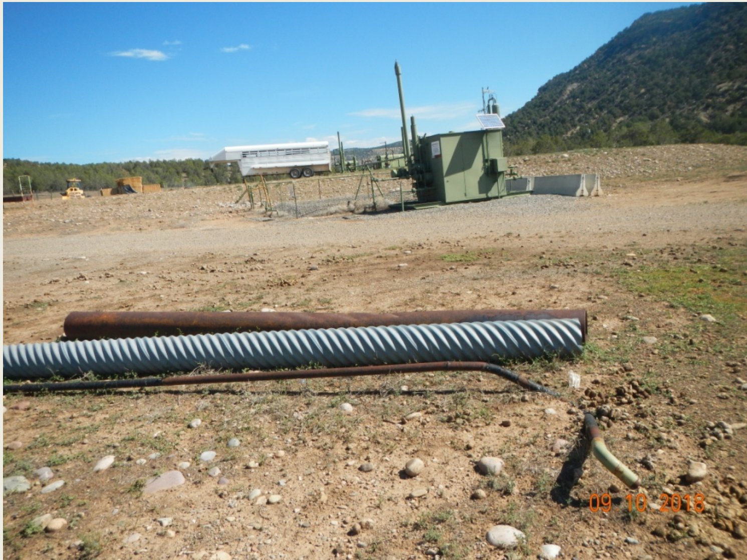
Photo 3. View of the western project area from the southwestern edge facing northward. Pipes need to be properly stored off of the well pad.
