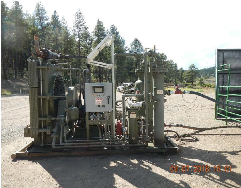
Skid mounted compressor.
