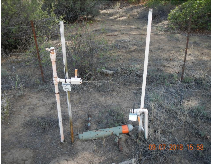
One inch risers on south side of location.
