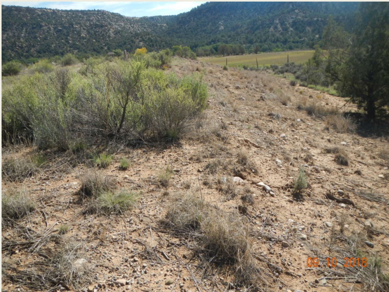
Photo 4. View of the southern fill slope from the southwestern edge facing eastward. Some rilling is occurring here as vegetation is more sparse on the slope.
